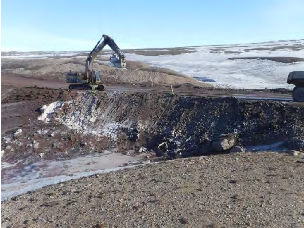
Photo 1. Snow clearing at the outlet of BG-01 on May 6, 2019
