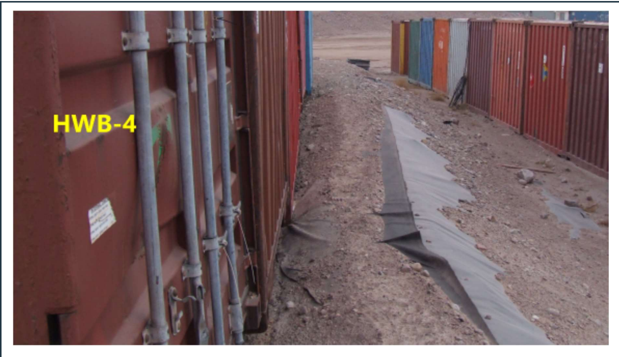
Figure 43: Perimeter berm at the HWB-4 cell, with exposed geotextile and liner.
