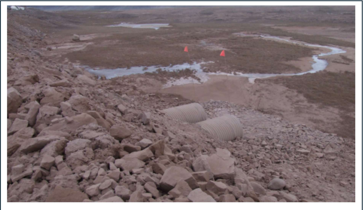
Figure 59: Water seepage through and beneath the road embankment near the tote road culverts.
