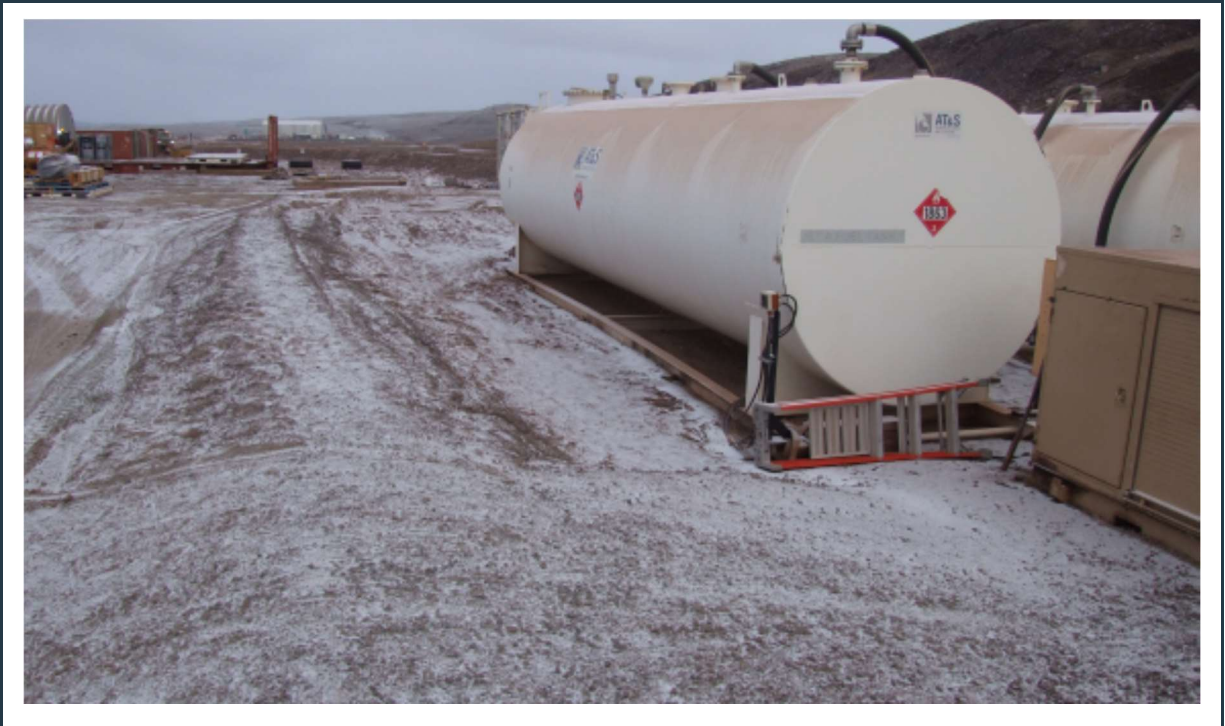
Figure 29: View of the berm around the jet fuel storage with two fuel tanks.
