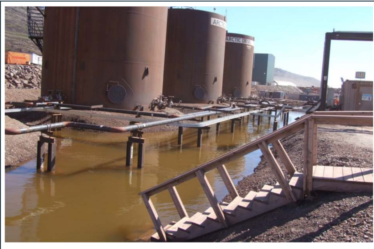
Figure 34: View of the MS-03 diesel fuel farm
