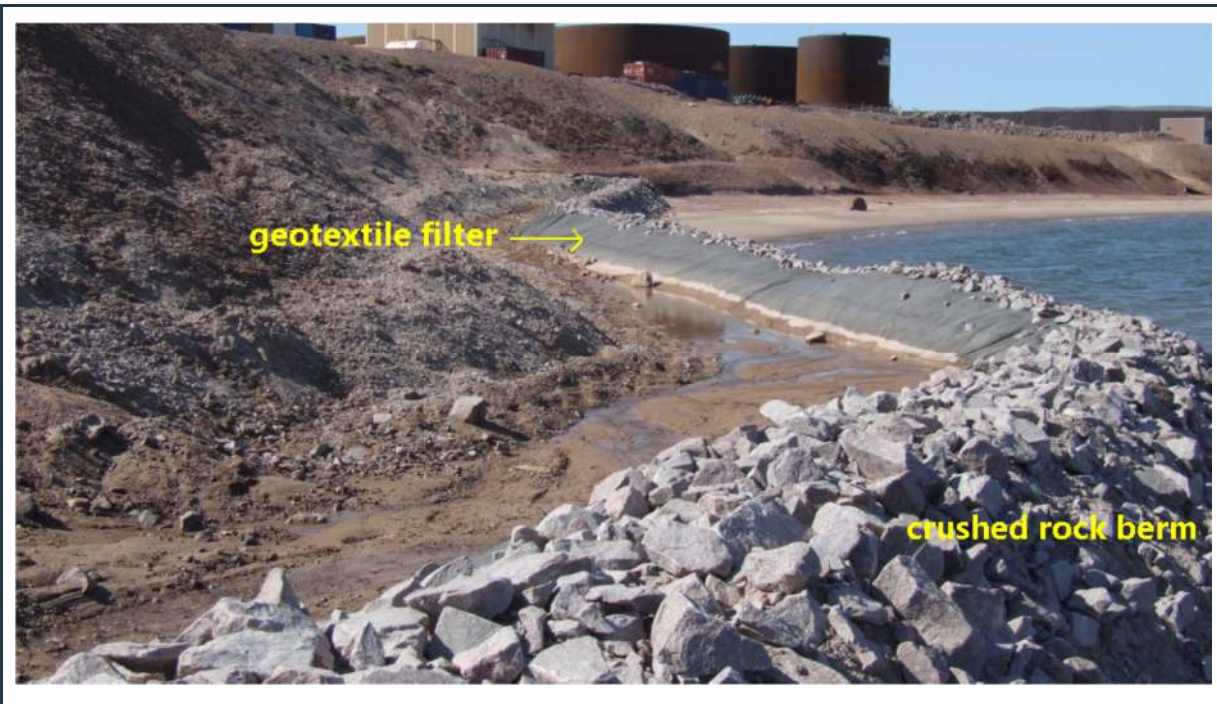
Figure 61: View of the freight dock check dam/berm with geotextile filter on the upstream face of the crushed rock berm, to retain silt
