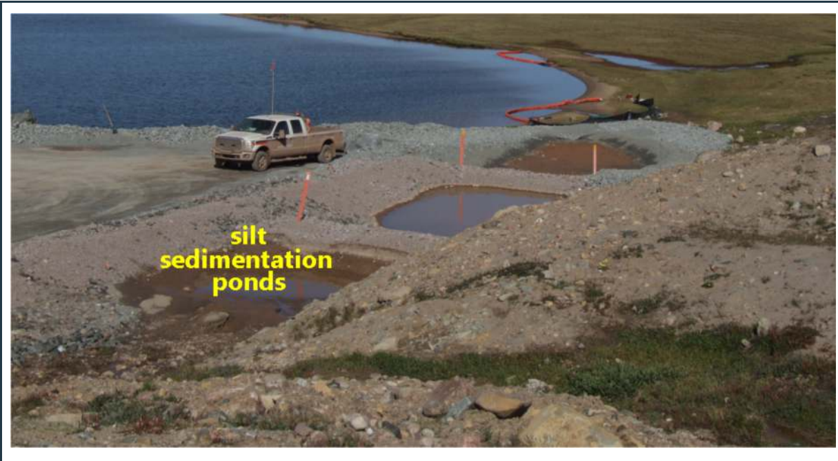
Figure 38: CLSP silt sedimentation check dams forming small ponds
