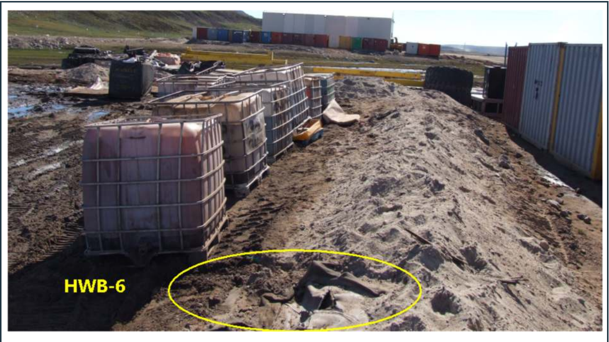
Figure 16: View of HWB-6. Note the damaged liner at the yellow circle.
