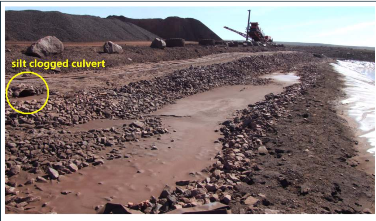
Figure 22: Surface water collection ditch with clogged culvert
