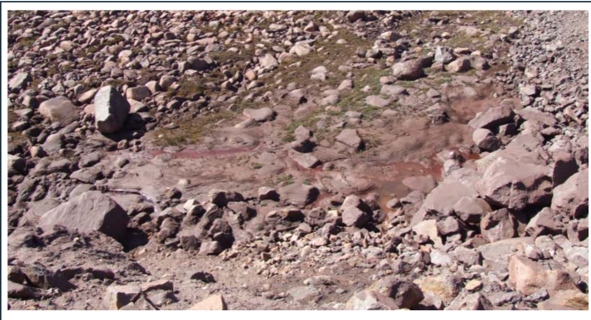
Figure 24: Water seepage at the toe of the tote road embankment near the crusher pad
