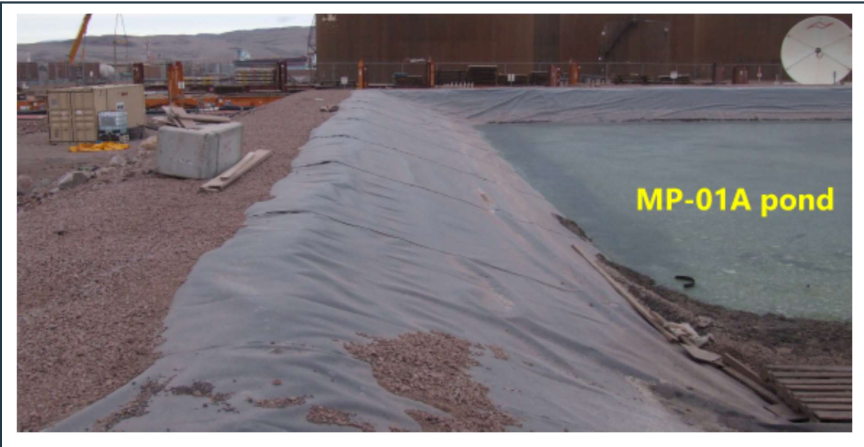
Figure 45: Berms and liner in good condition, with stable slopes around the MP-01A pond.
