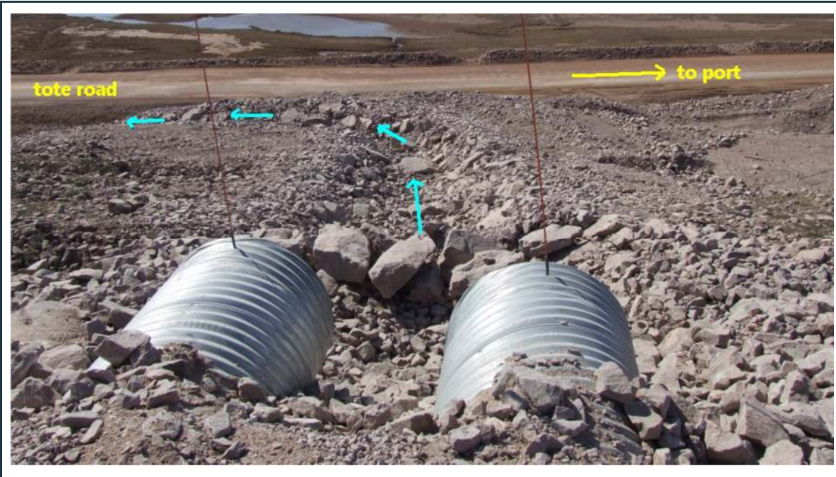
Figure 68: Culverts and drainage ditch, conveying surface water from higher elevation toward the road
