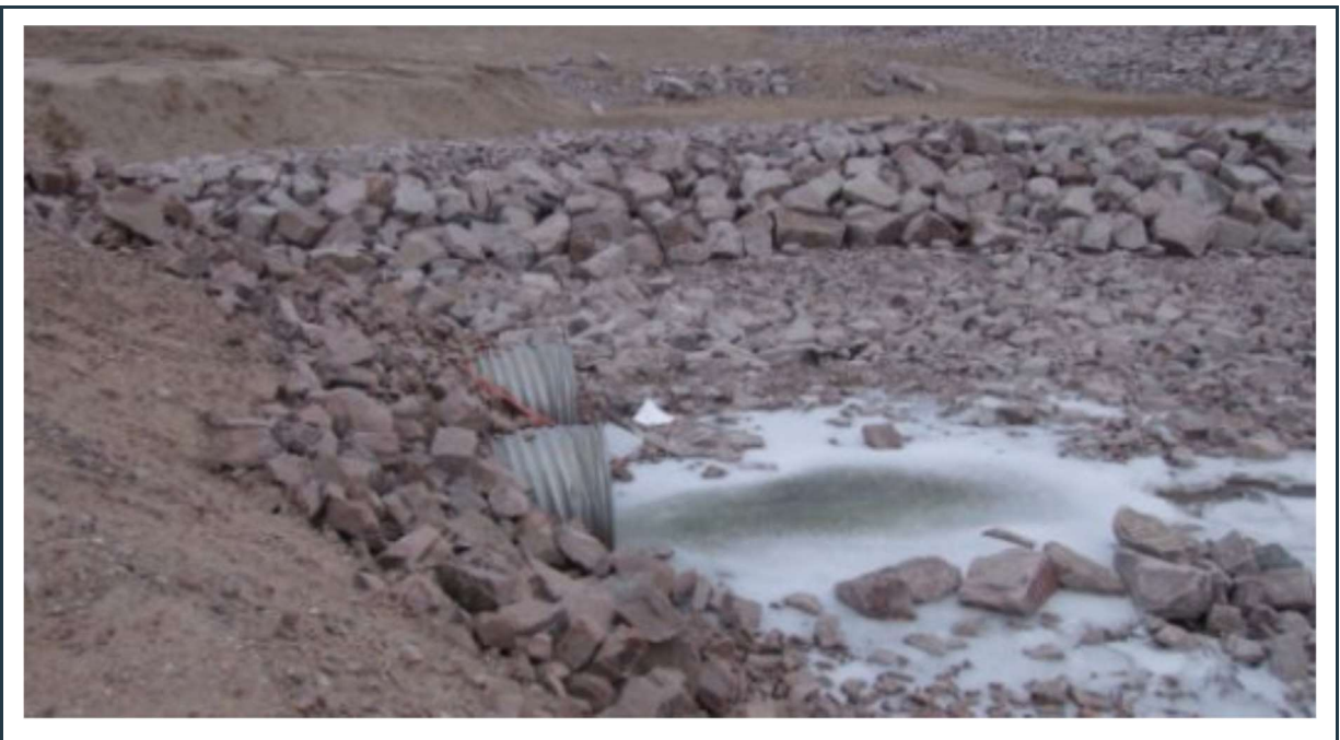
Figure 56: View of the P-SWD-7 surface water collection ditch and culverts, adjacent to the new freight dock (under construction).
