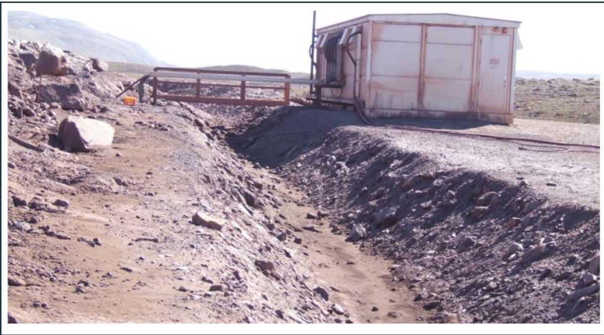
Figure 21: Surface water collection ditch around the crusher plant
