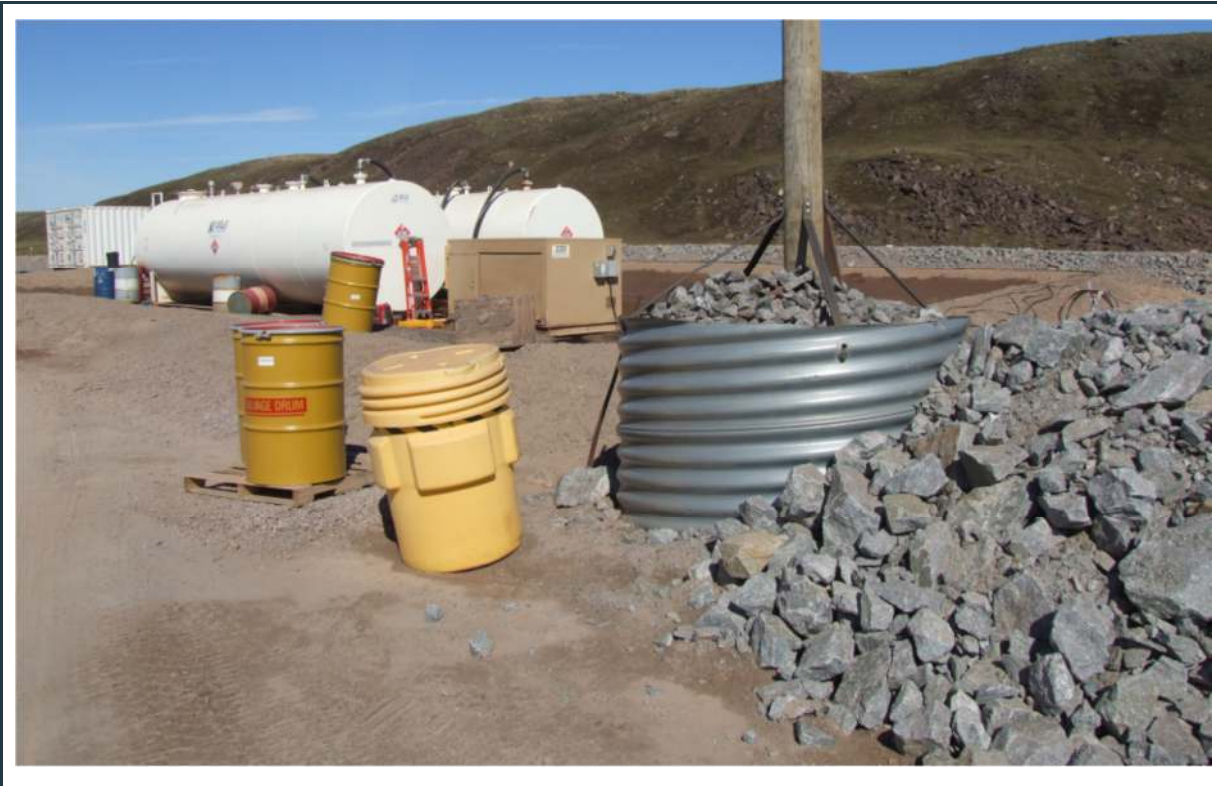
Figure 32: View of the jetfuel farm's double berm system (note the additional crushed rock berm)
