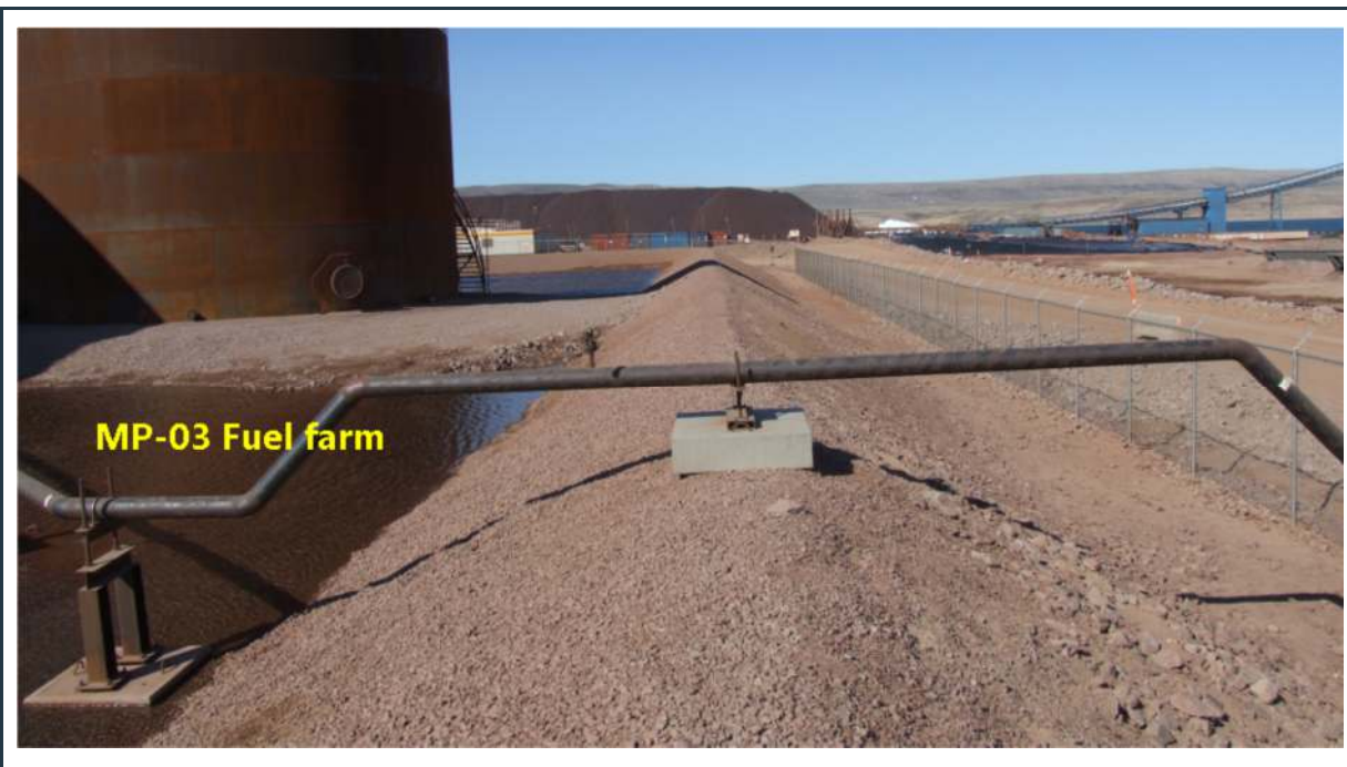
Figure 51: View of stable, well maintained berms around the MP-03 fuel tank farm
