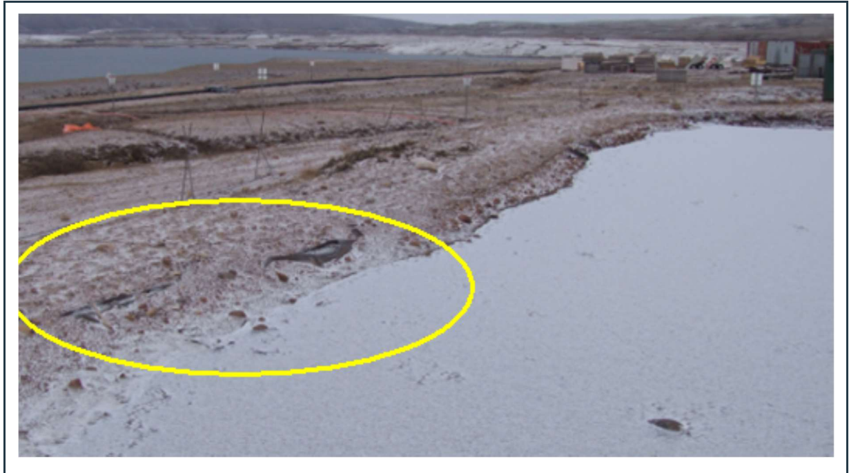
Figure 27: View of the locally low generator berm (high water level with frozen surface).
