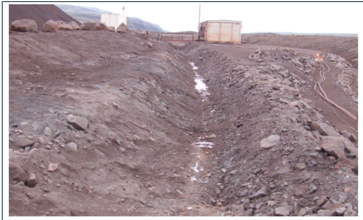
Figure 18: Surface water collection ditch around the crusher plant.
