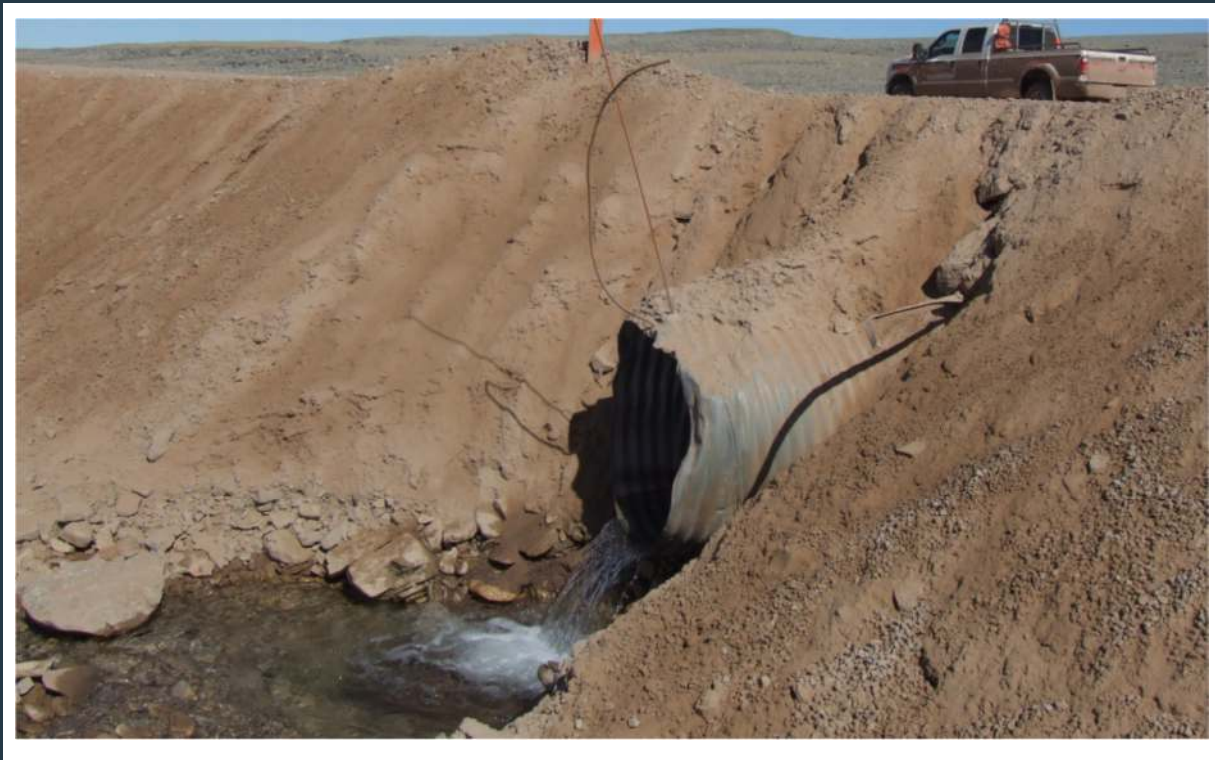
Figure 86: View of culvert 083 (outlet) with some slope erosion
