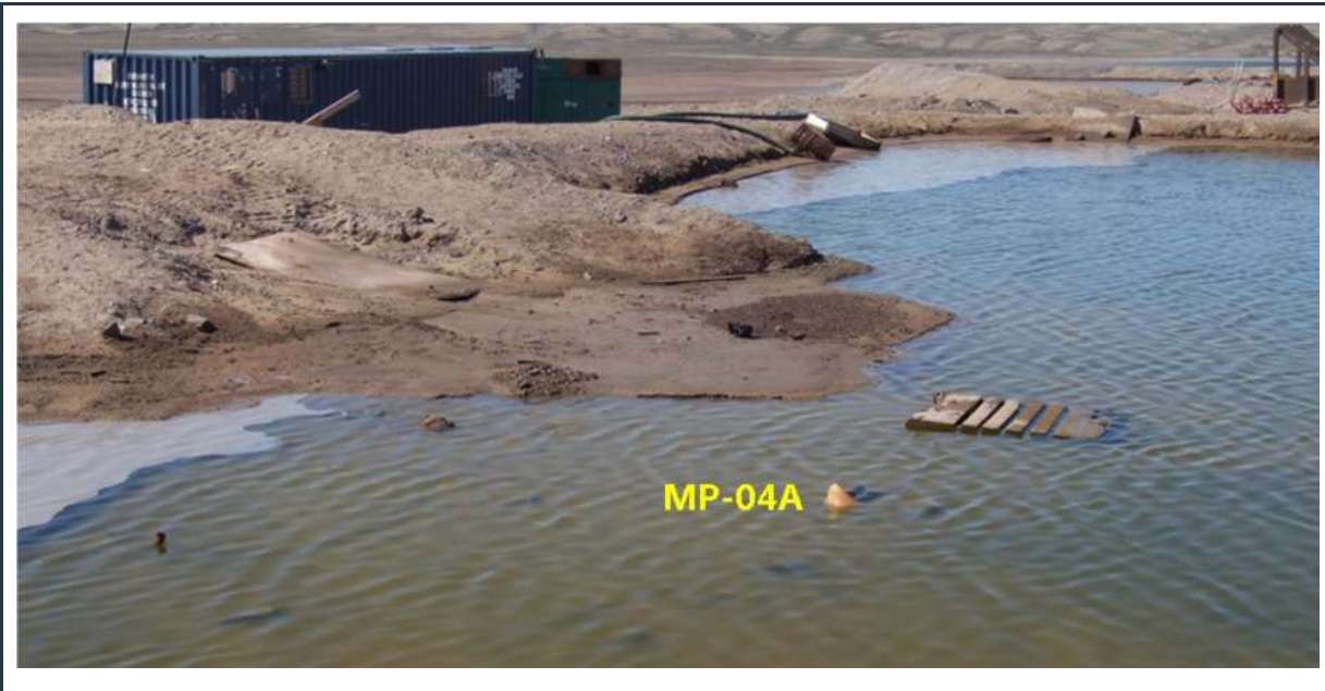
Figure 54: Condition of the ramp at the MP-04A contaminated snow dump
