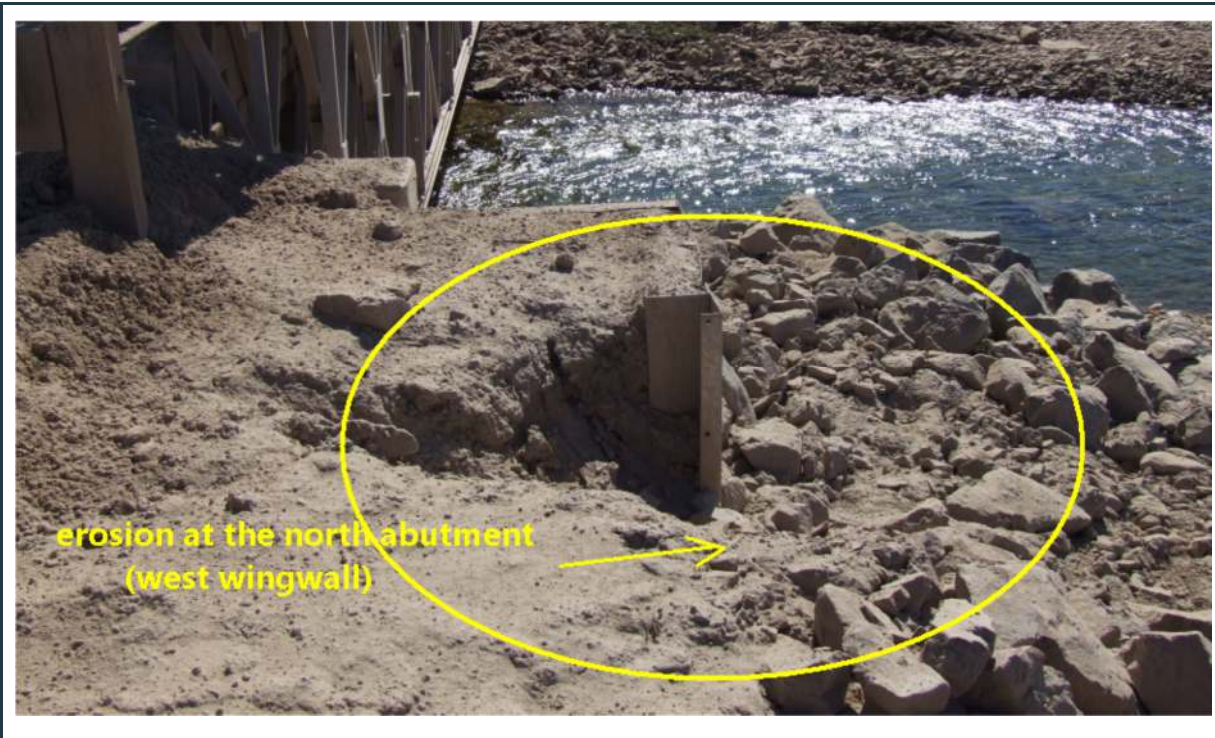
Figure 78: Minor erosion at the north-west wingwall at bridge 63
