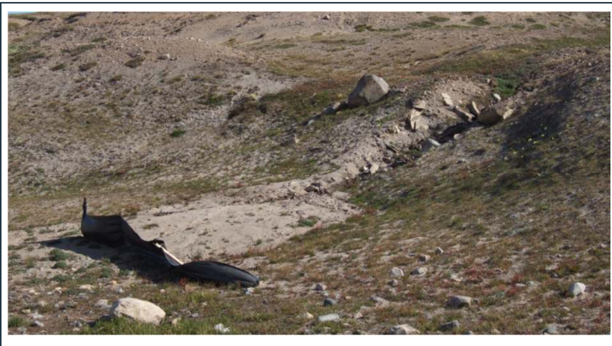
Figure 39: Slope erosion in the vicinity of the CLSP check dams
