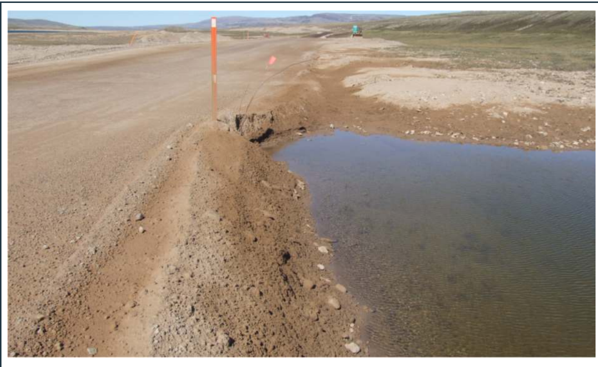
Figure 93: View of culvert 107 (inlet). Extension of the culvert is required.
