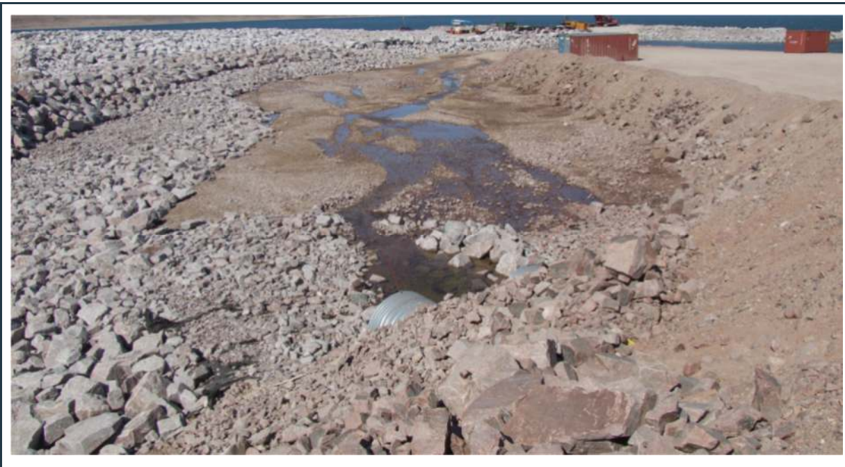
Figure 65: P-SWD-7 surface water collection ditch adjacent to the new freight dock (under construction)
