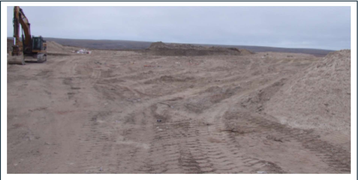
Figure 34: Solid waste disposal facility (waste continuously covered with clean soil fill).
