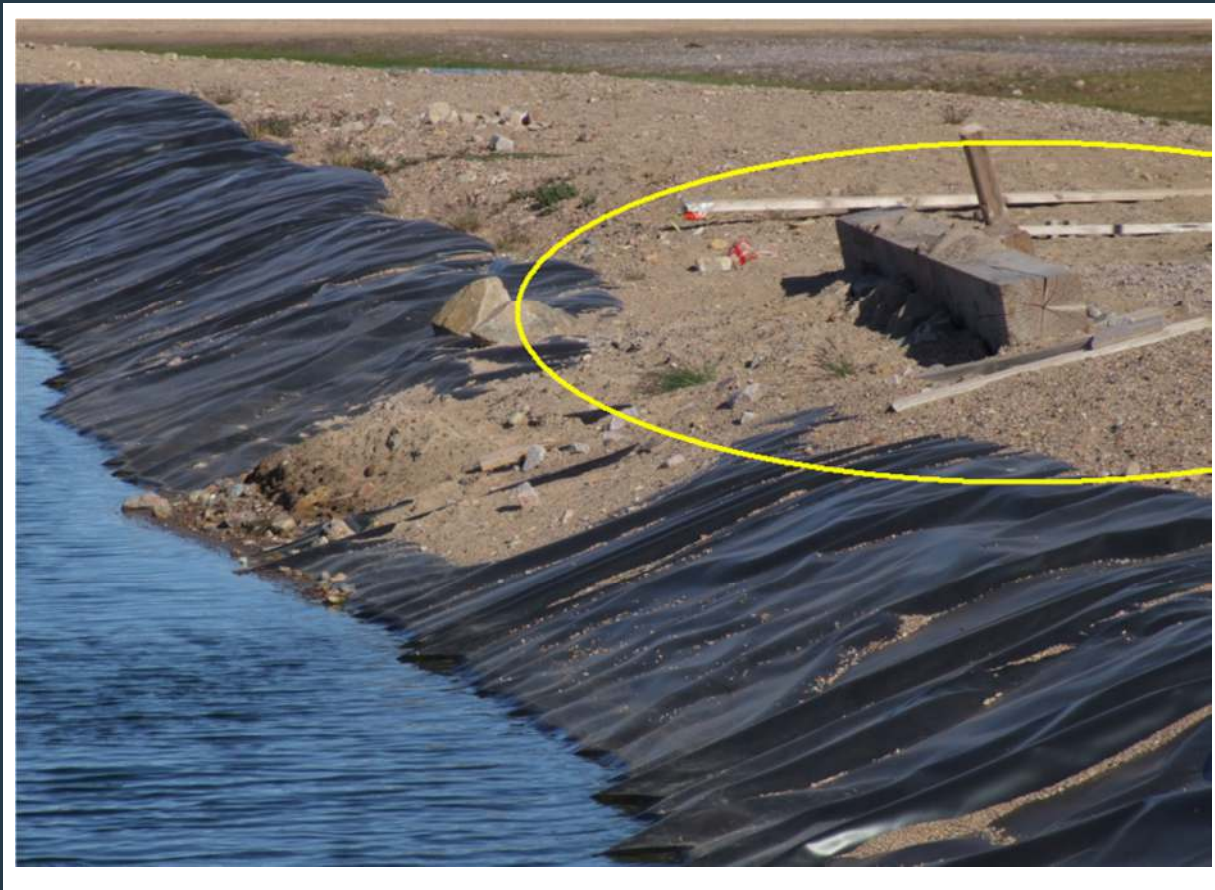
Figure 8: PWS pond #2 – Lower crest elevation caused by truck traffic at the water discharge point (yellow circle)
