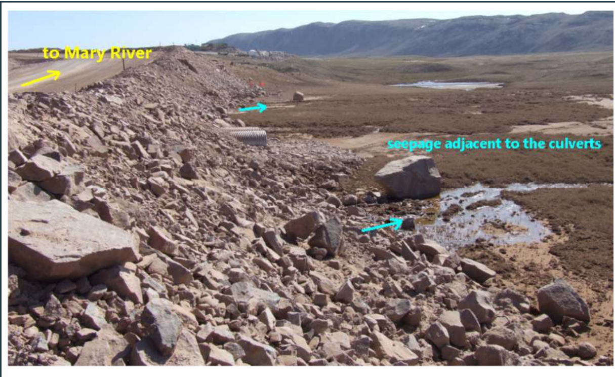
Figure 70: Water seepage through the road embankment adjacent to the tote road culverts
