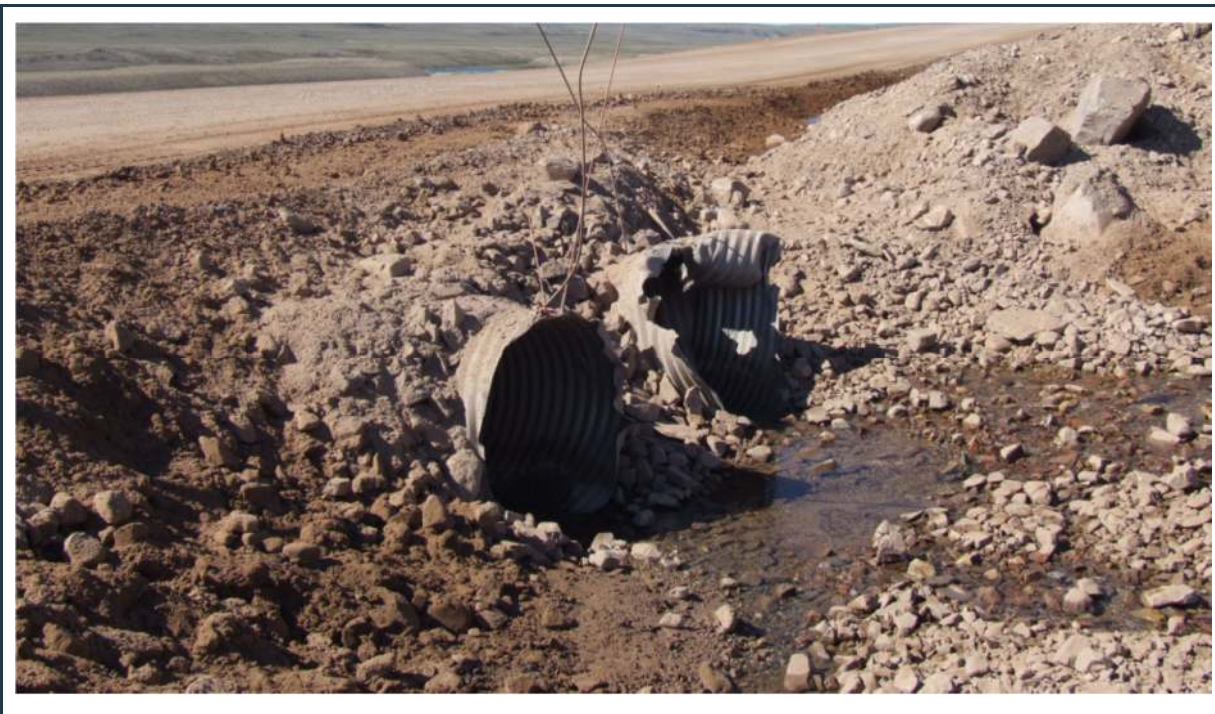
Figure 101: View of culvert(s) 114D (somewhat damaged inlet). Repair is required.
