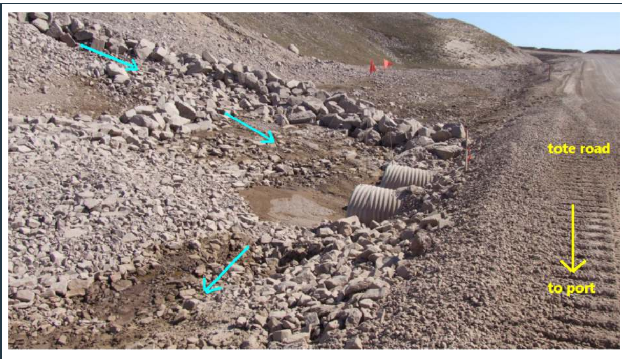
Figure 69: Surface water bypassing the two culverts installed under the tote road
