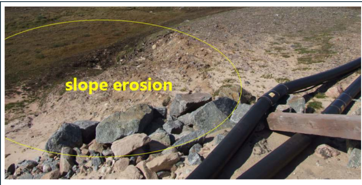
Figure 41: Minor slope erosion adjacent to the water discharge area.
