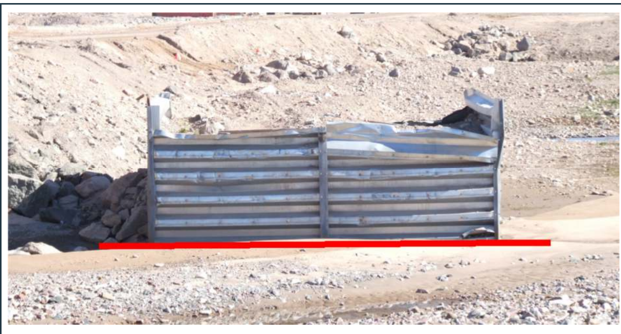
Figure 81: One of the "old" abutments at bridge 97. The section above the red-line may be removed, but the removal is not necessary.
