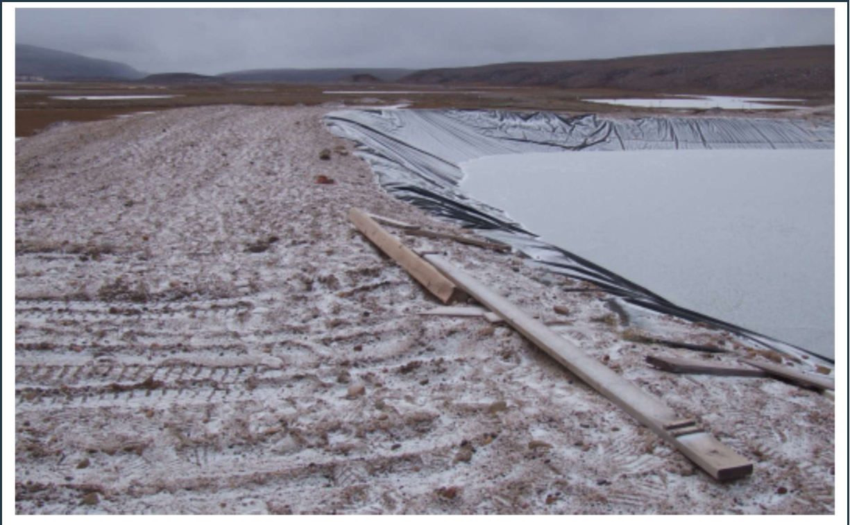
Figure 7: PWS pond #3 – Timber/lumber debris visible on the crest that should be removed.
