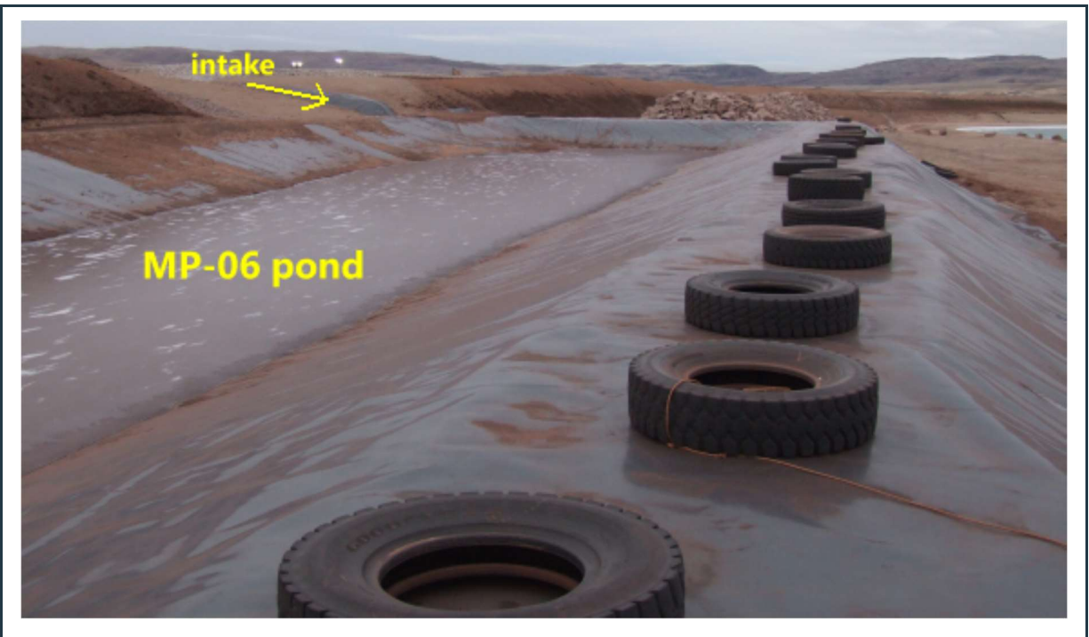
Figure 52: View of the MP-06 pond at the front of the north-west corner of the ore stockpile.
