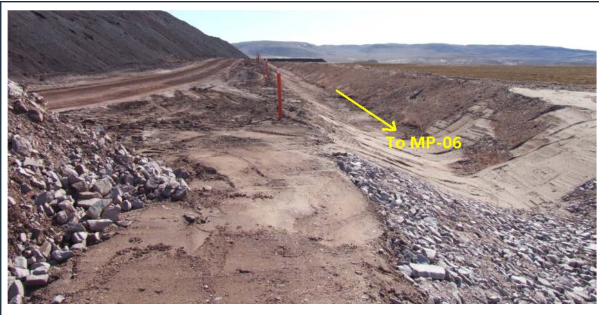
Figure 60: Surface water collection ditch, adjacent to stored, crushed ore leading to the MP-06 pond
