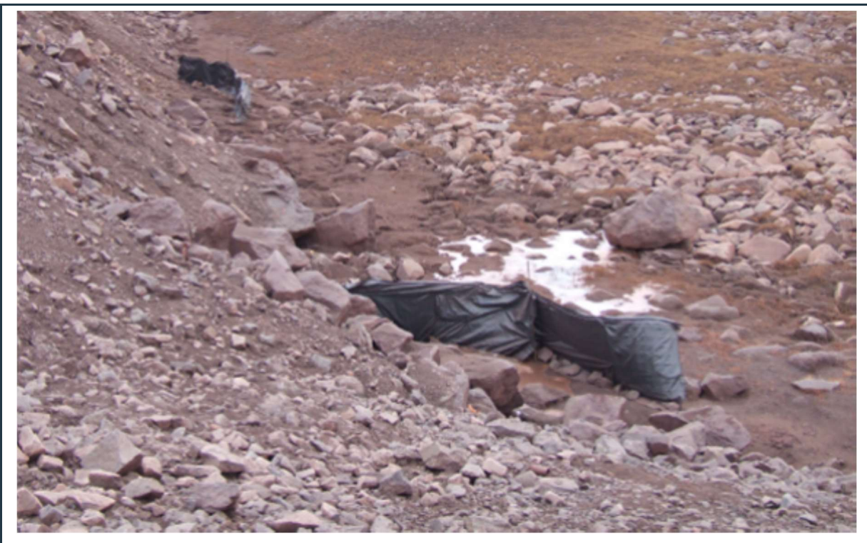
Figure 20: Minor water seepage as ice mount at the toe of the embankment where the crusher pad ditch embankment fill meets the tundra.
