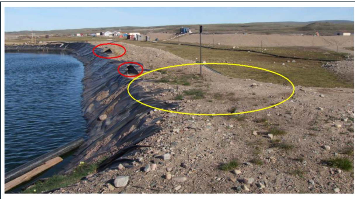
Figure 7: PWS pond #1 – Lower crest elevation (yellow circle) and damages to the liner (red circles)
