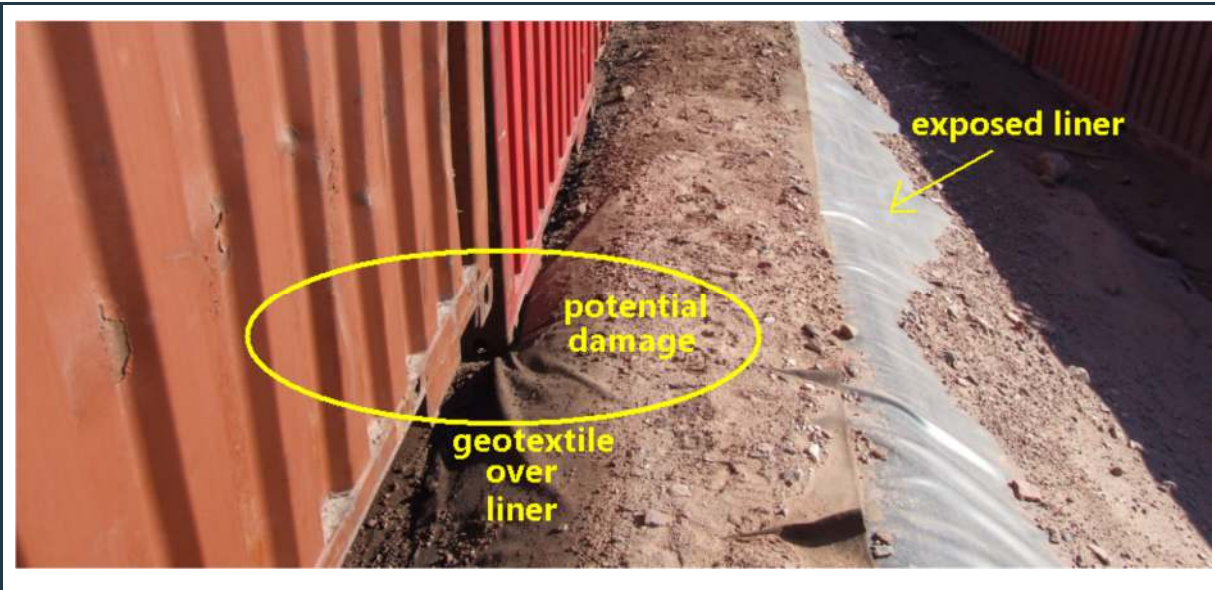
Figure 48: Exposed geotextile and liner at the HWB-4 pond, with location of potential damage to liner
