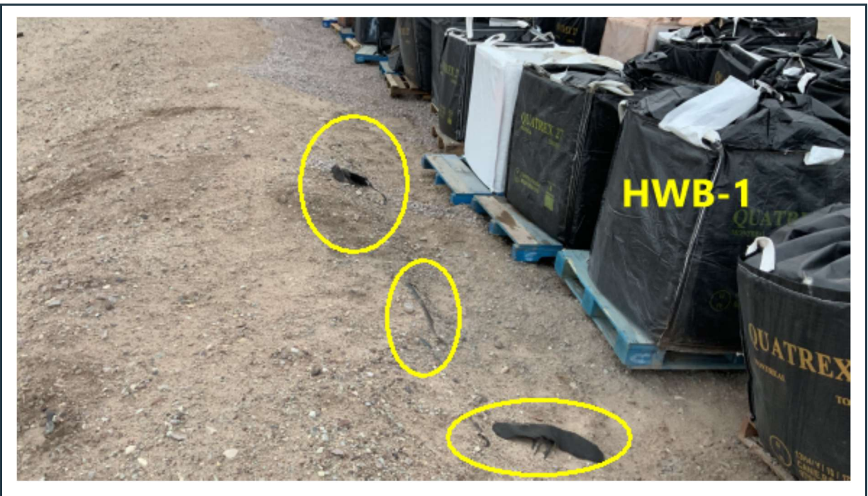
Figure 40: Ripped geotextile and exposed liner at the stable northern berm of the HWB-1 cell.
