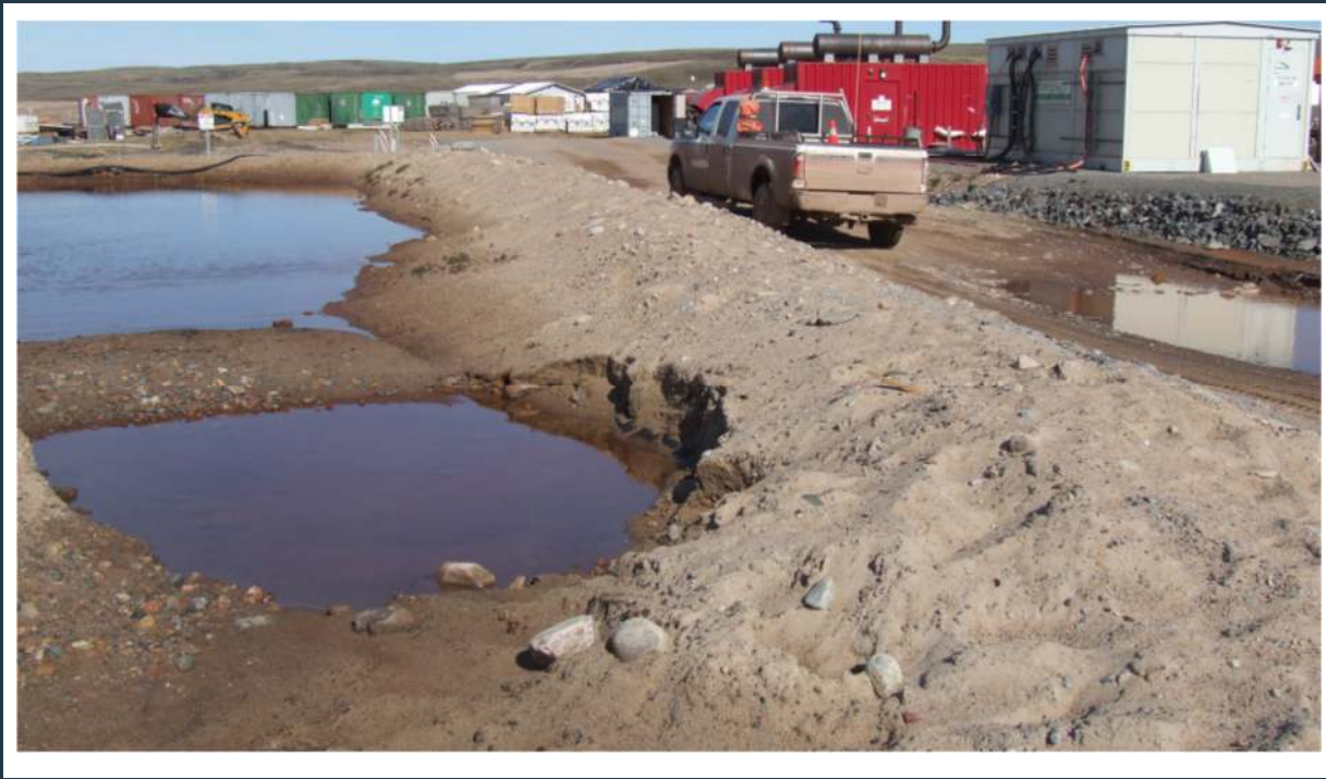
Figure 30: View of minor slope problem at the south-east corner of the berm at the Genset pond
