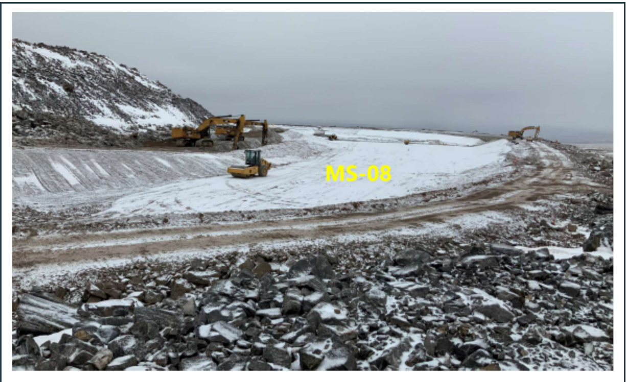
Figure 24: Construction of the new MS-08 pond, immediately adjacent to the waste rock dump.
