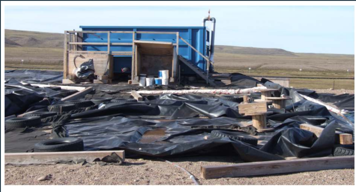
Figure 10: PWSP #2 and #3 – Untidy conditions at the water discharge point between ponds #2 and #3
