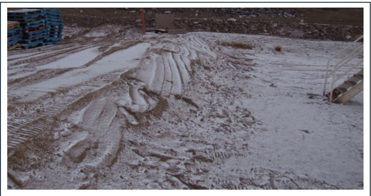
Figure 30: Recently placed granular fill on the berm's crest, to protect the previously exposed liner.
