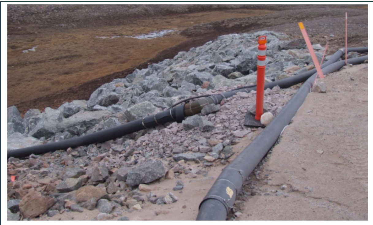
Figure 38: Recently stabilized slope erosion adjacent to the water (effluent) discharge site.
