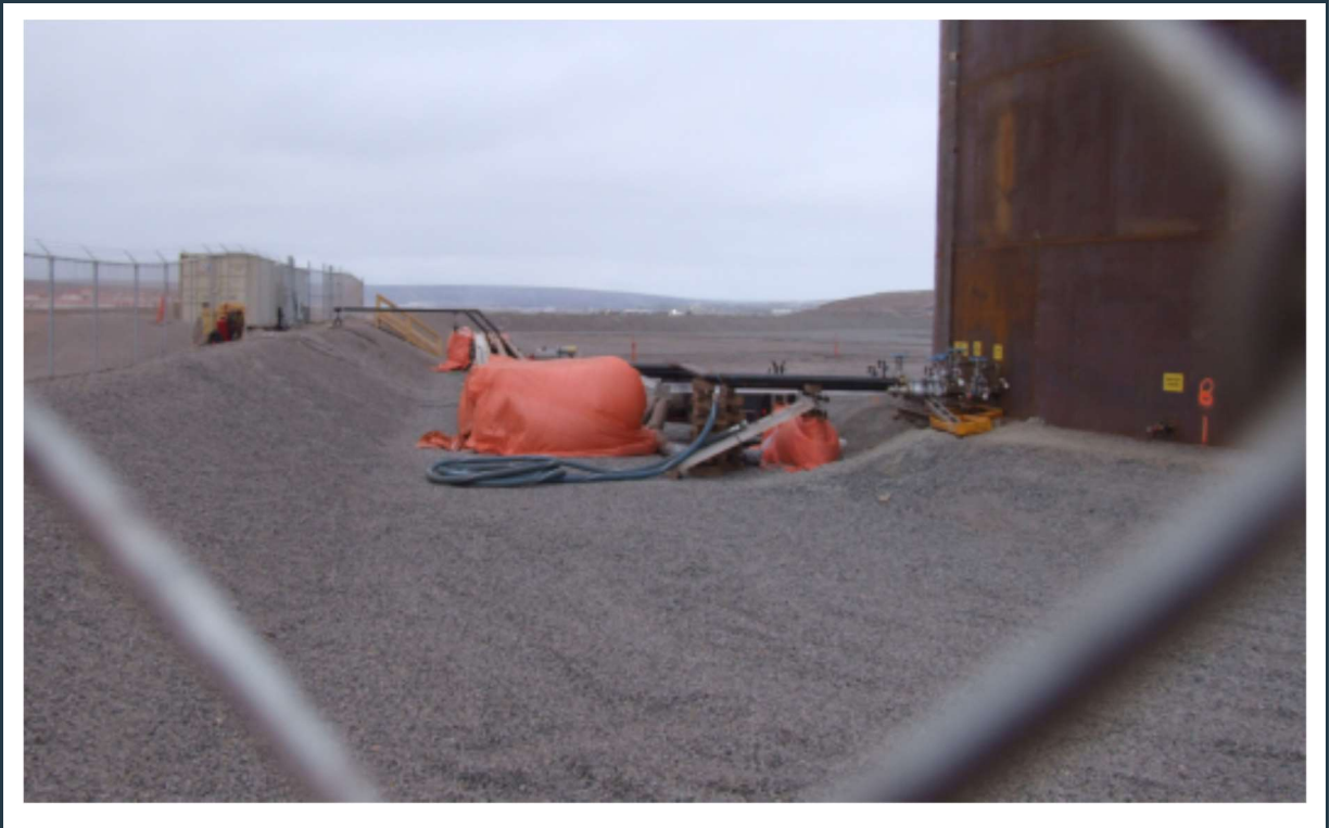
Figure 33: View of the recently completed new fuel storage at the Mary River site.
