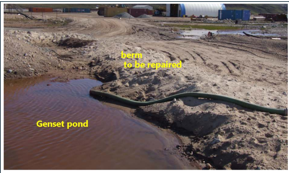
Figure 31: View of the south section of the berm that needs to be repaired (raised and regraded)
