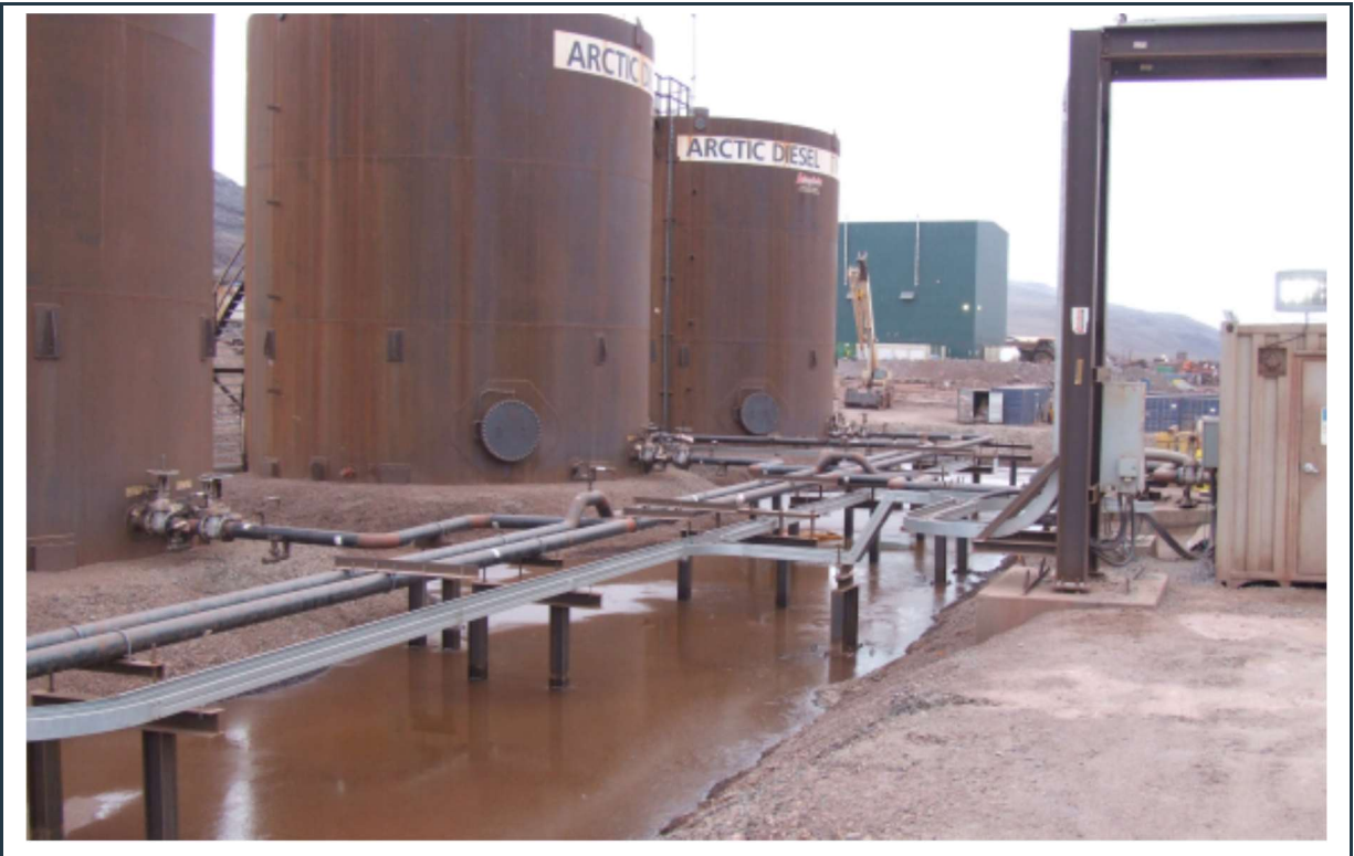
Figure 31: View of the MS-03 diesel fuel storage with frozen water surface.
