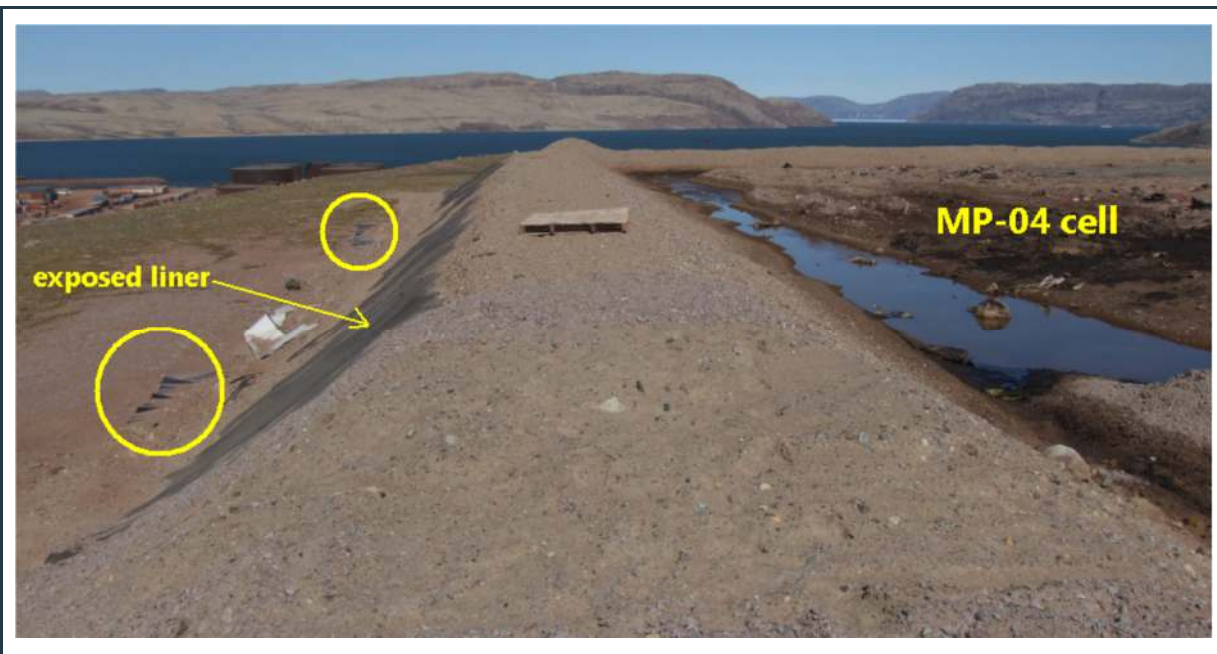
Figure 53: Stable berm at the MP-04 landfarm with exposed liner on the downstream face of the berm
