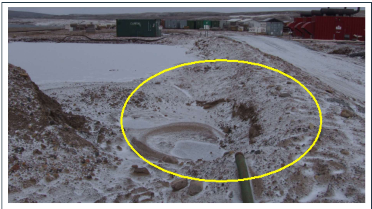
Figure 28: View of minor slope problem at the south-east corner of the generator berm.
