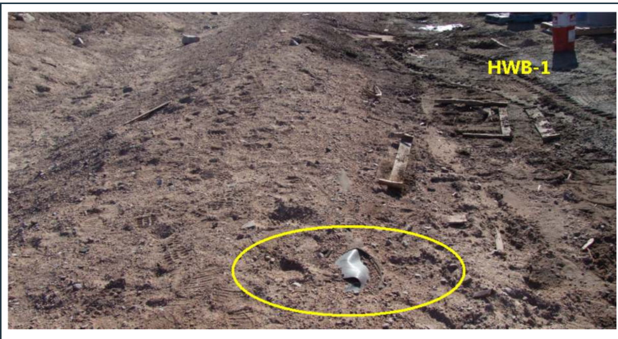
Figure 43: Ripped geotextile and exposed liner at the HWB-1 cell
