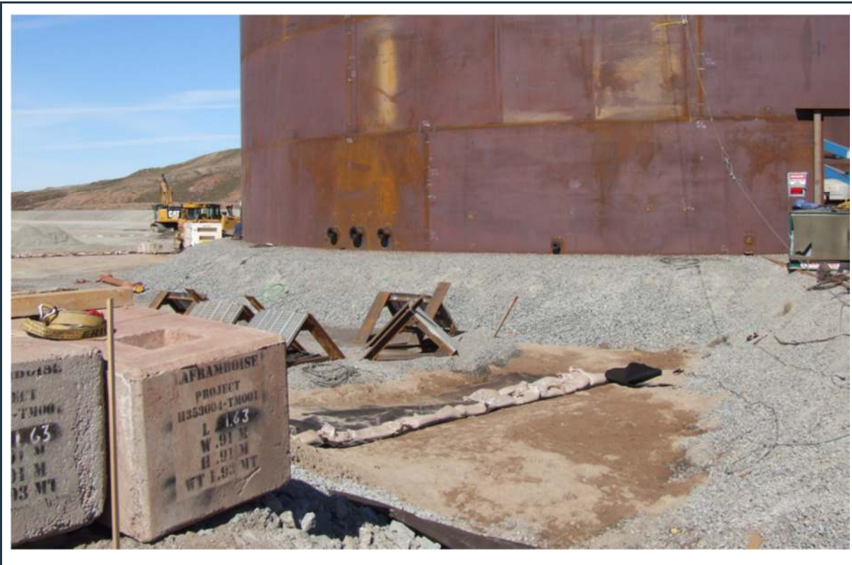
Figure 36: View of the new fuel tank farm at the Mary River site (under construction)
