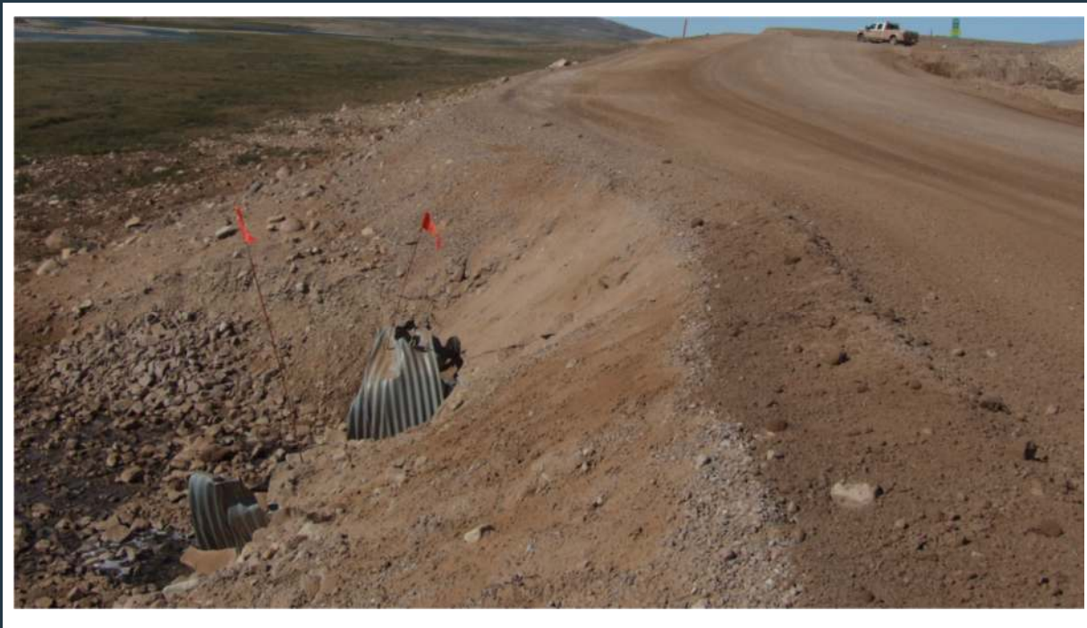
Figure 100: View of culvert(s) 114D (somewhat damaged outlet). Repair and extension is required.
