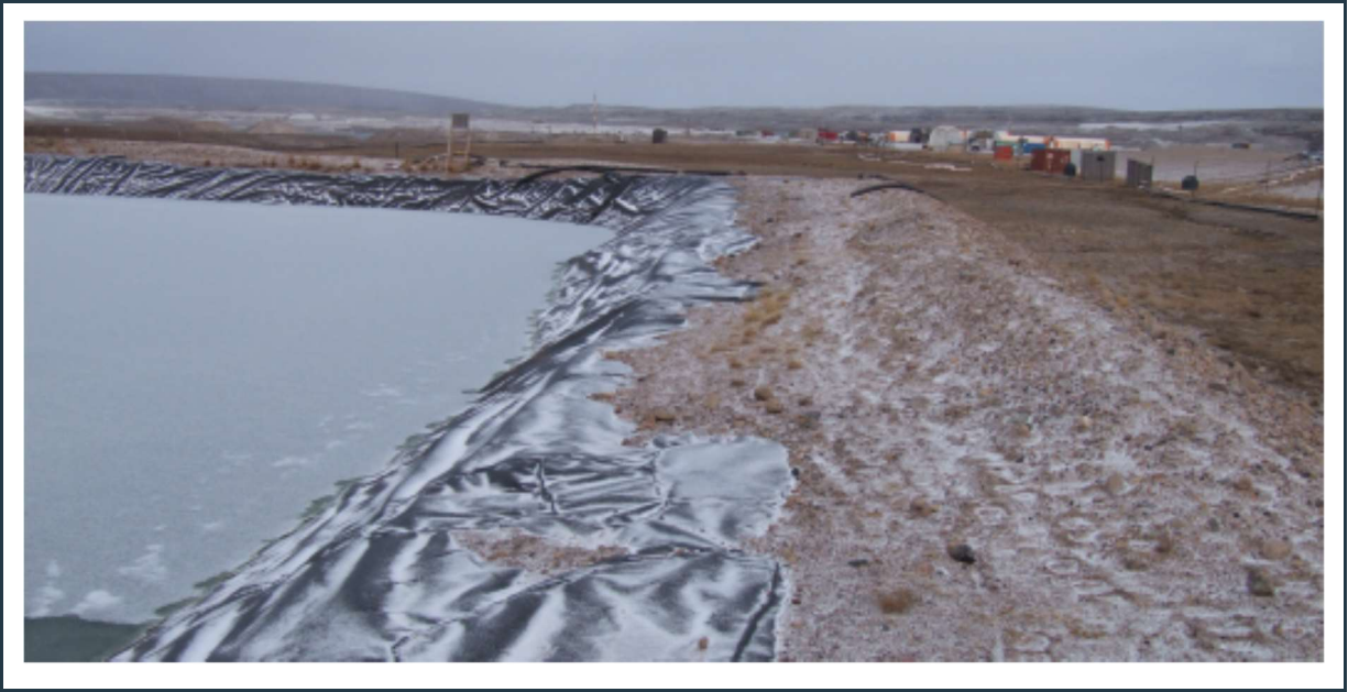
Figure 5: PWS pond #1 – View of repaired liner and additional fill on the berm's crest.
