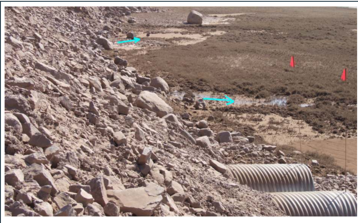
Figure 71: Water seepage through the road embankment adjacent to the tote road culverts
