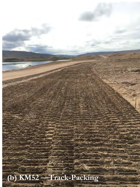
Photo 6. KM52 — Rough and loose (a) and track-packing (b).
