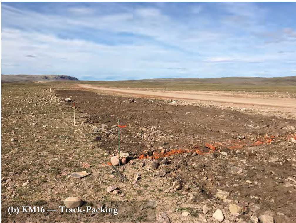
Photo 7. KM16 — Rough and loose (a) and Track-Packing (b).
