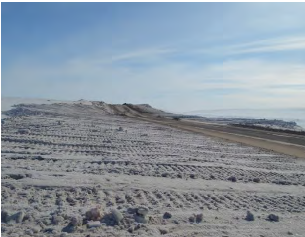
Photo 13 Example of snow bank management on east and west sides of Tote Rd to ensure they do not exceed the maximum snow depth at km 28, April 21, 2017.
