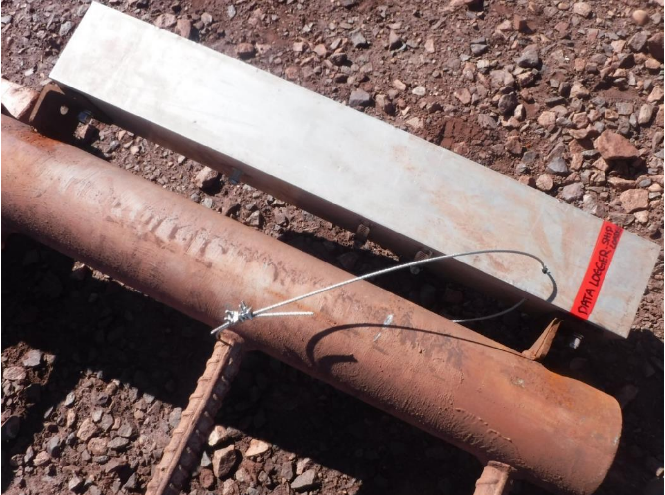
Figure 2: Hardware attaching aluminum tube to steel L brackets and wire rope for redundancy of the L bracket attachments.
