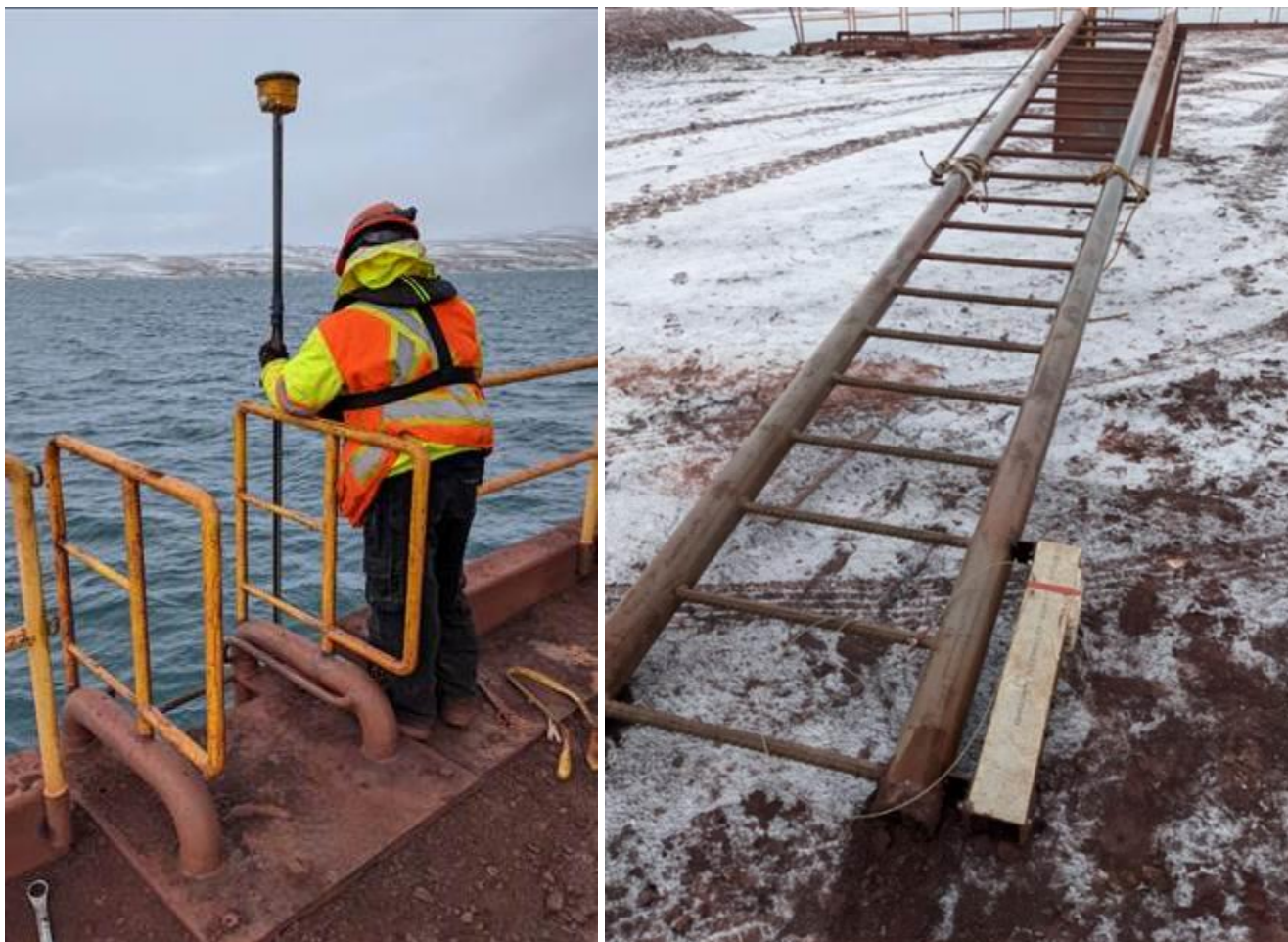
Figure 1: Left: RTK Survey of the ore dock ladder top plate. Right: Ore dock ladder following removal, with the tide gauge housing shown on the bottom right of the ladder. (Ritgen, 2020)
