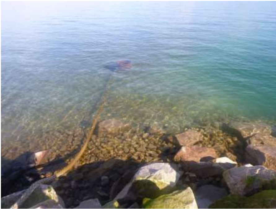
Photo 3: North side of Freight Dock, looking north during site visit on 7 August 2020 at 0.4 m tide. Water depth approx. -1.0 m CD. Submerged cut steel pile offshore of offset habitat.
