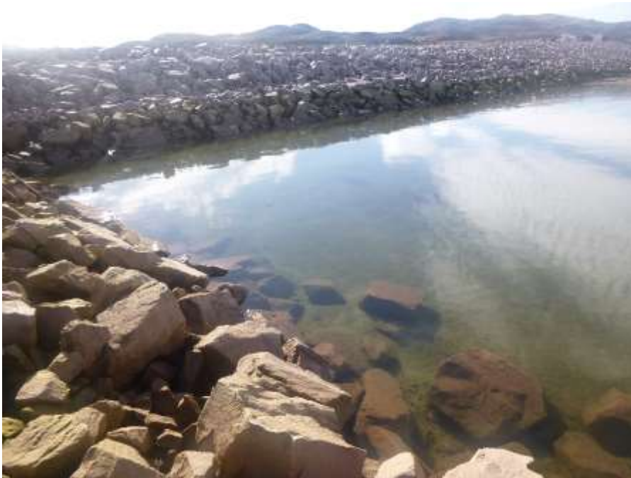
Photo 1: West side of Freight Dock, looking southeast, during site visit on 7 August 2020 at 0.4 m tide. Intertidal and upper subtidal extending to the sand beach (approx. water depth: -0.1 to -0.4 m below chart datum (CD)). Green filamentous algae observed in intertidal. A school of larval fish (approx. 50 individuals) observed in area of riprap substrate.
