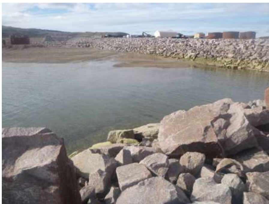
Photo 8: East side of Freight Dock, looking south during site visit on 7 August 2020 at 0.4 m tide. Green filamentous algae observed on riprap armouring in intertidal/upper subtidal. Freshwater source observed center-left of photo. Water depth along causeway was approx. -0.1 to -0.8 m CD.
