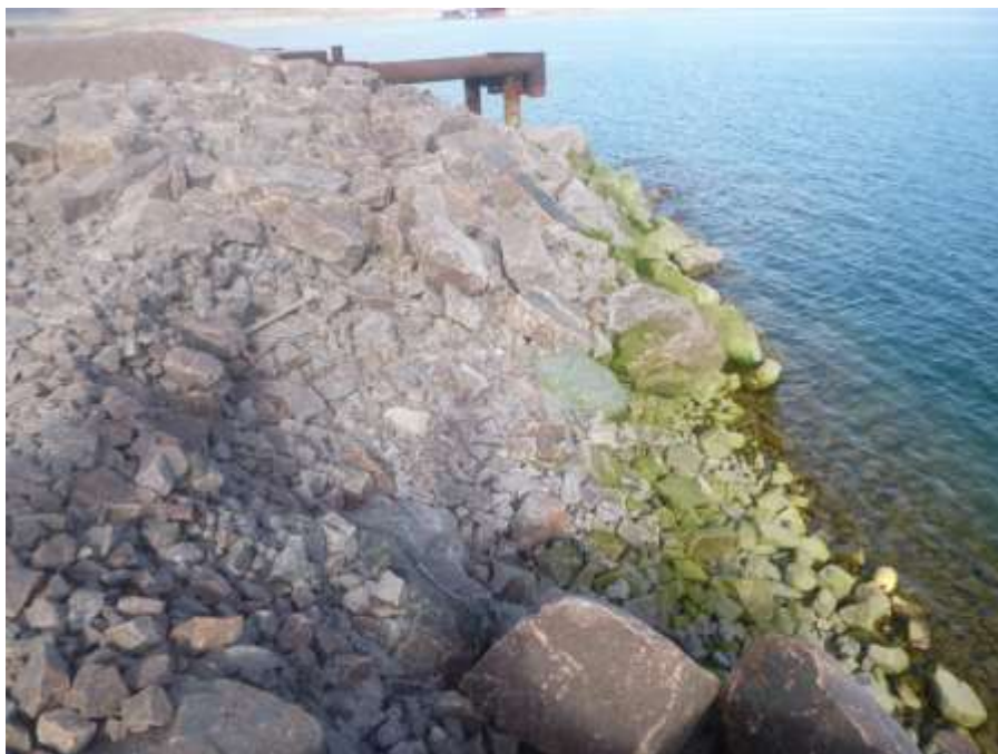
Photo 5: North side of Freight Dock, looking northwest during site visit on 7 August 2020. Section (3 m wide) of exposed crushed rockfill with minimal rock armouring.
