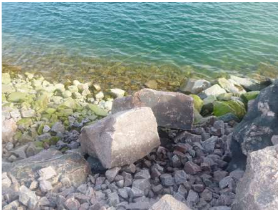
Photo 6: North side of Freight Dock, looking north during site visit on 7 August 2020. Alternate view of same section described in Photo 7, above.
