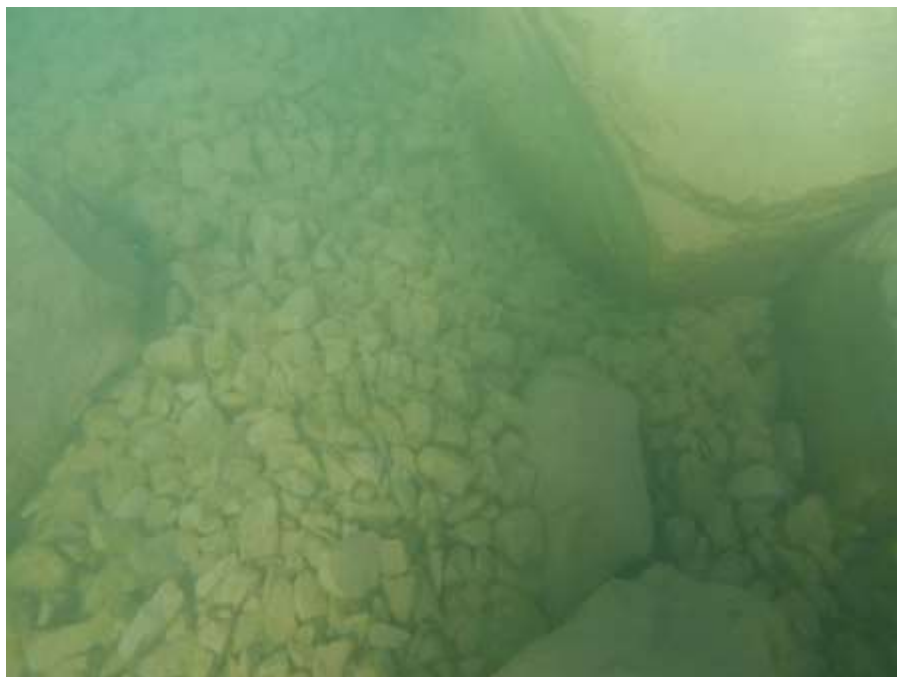
Photo 7: Exposed crushed rockfill in upper subtidal area, offshore of the north face of Freight Dock identified in Photo 5 and 6 (14 August 2020).
