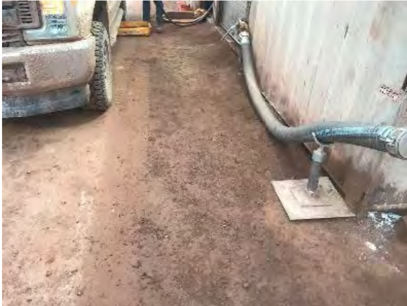
Photo 58: Site Reconnaissance at Fuel Farm MS03B, showing staining on the surface in fueling locations. September 27, 2021
