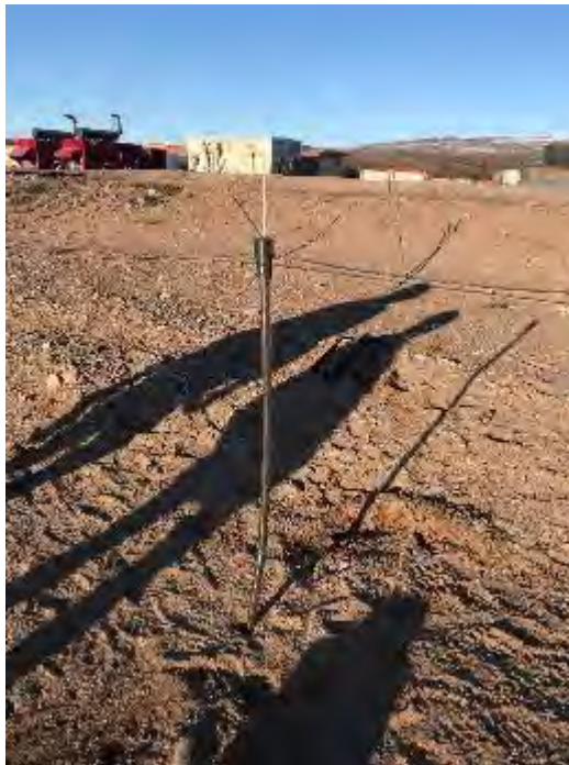
Photo 11: Attempted installation of drive-point piezometer at monitoring location MS-HWB-GW8, facing northwest. September 22, 2021
