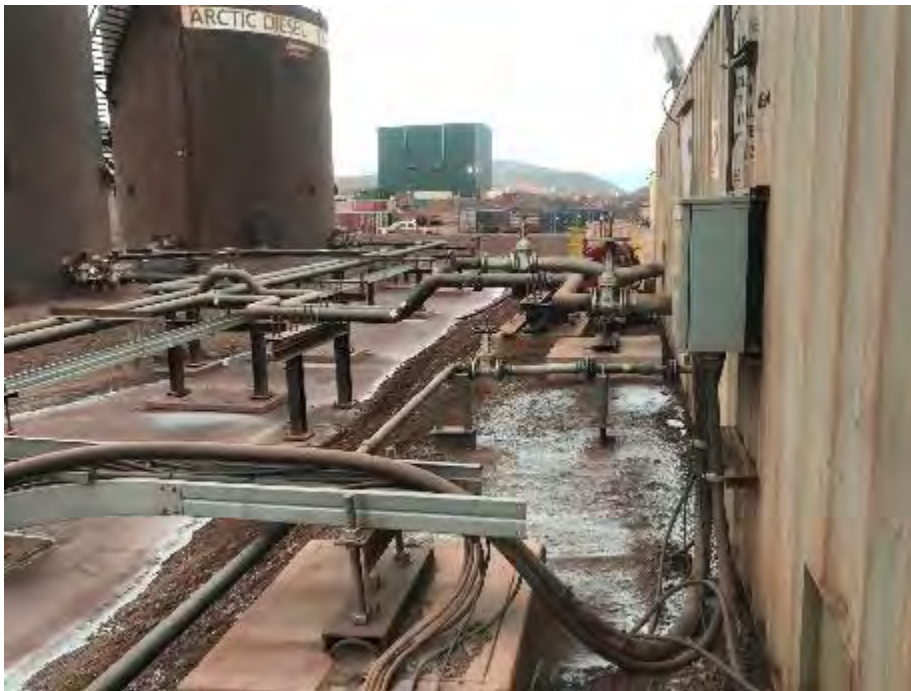
Photo 53: Site Reconnaissance at Fuel Farm MS03B showing pipe infrastructure. September 27, 2021
