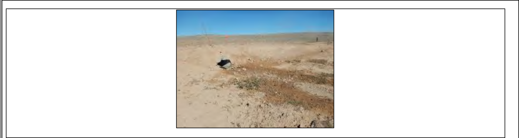
Photos 1. Photograph of the Tote Road crossing CV-086 from downstream looking upstream.
