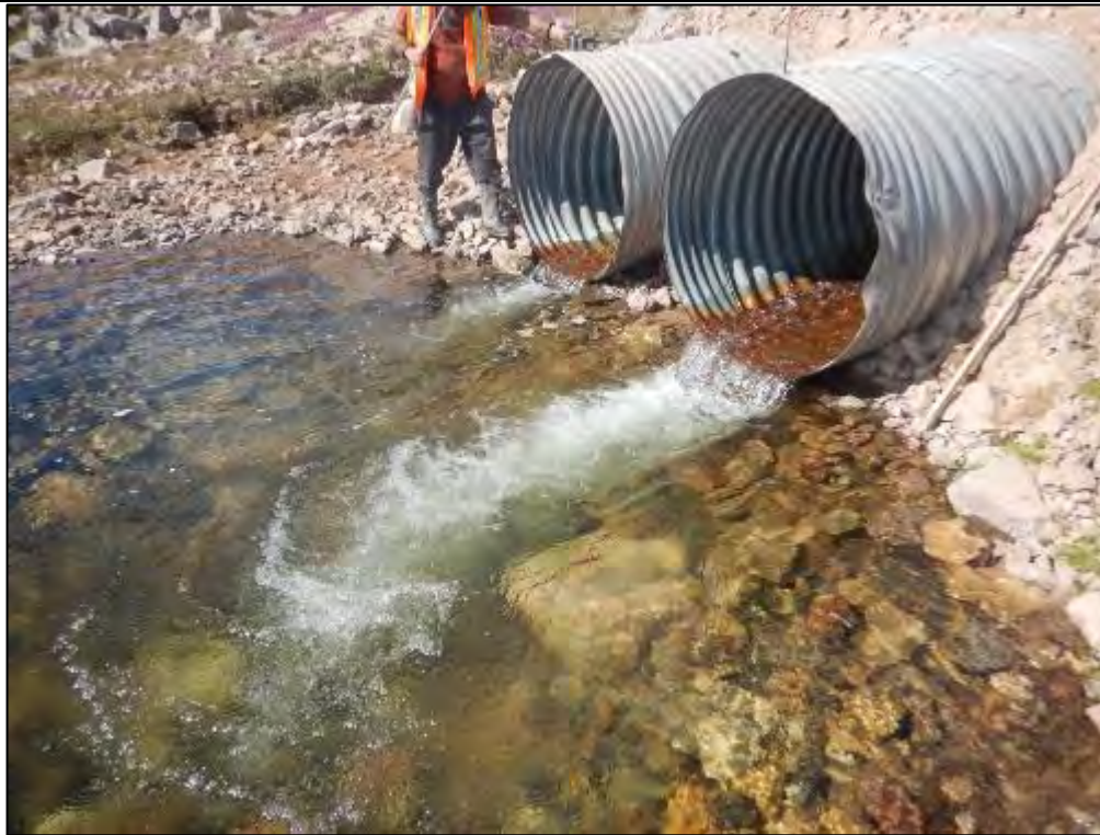
Photos 8: Photograph of the downstream end the perched culvert before remediation at CV-225. Remediation could not be completed in 2019.
