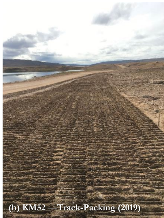
Photo 10. KM52 — Rough-and-loose (a) and track-packing (b).
